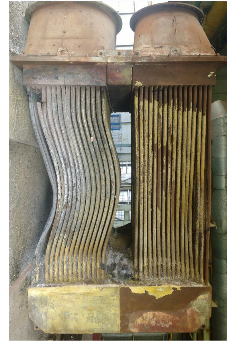
Heat exchanger after 12 years operation
